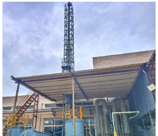
Thione Alkali Scrubber with Stack
