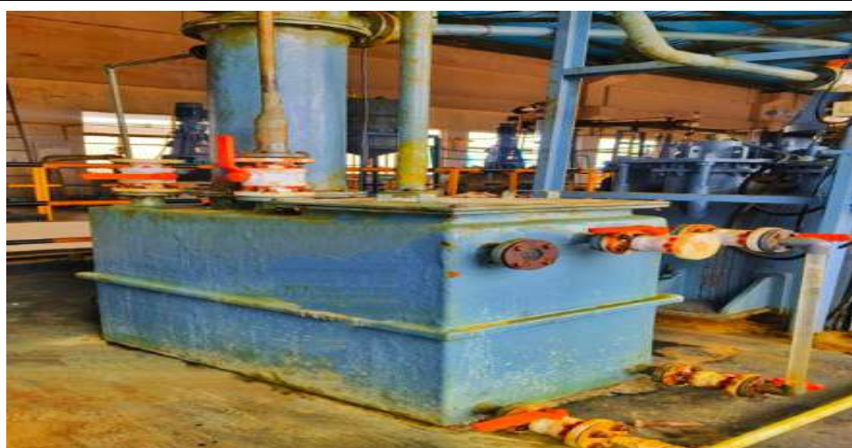
Alkali Circulation system for chlorine safety
