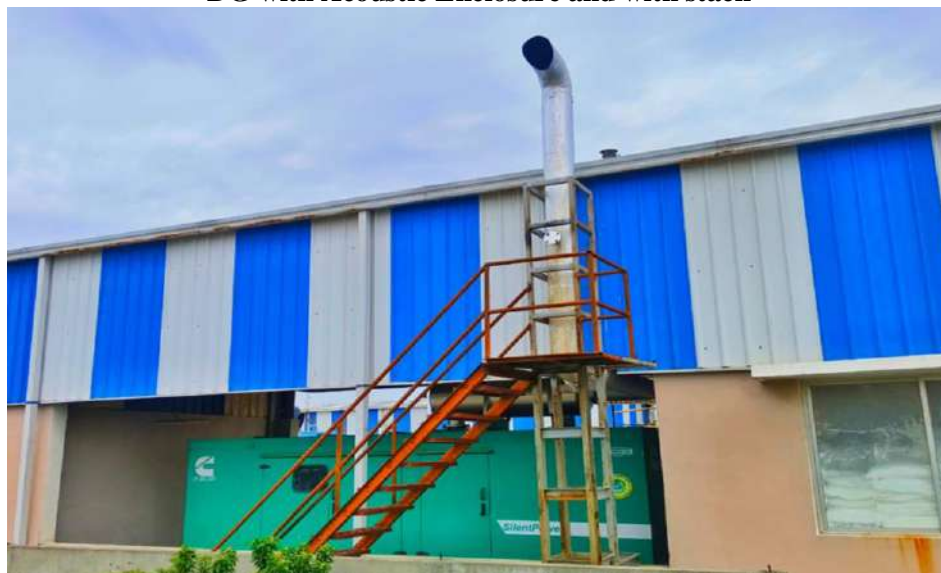
DG with Acoustic Enclosure and with stack
