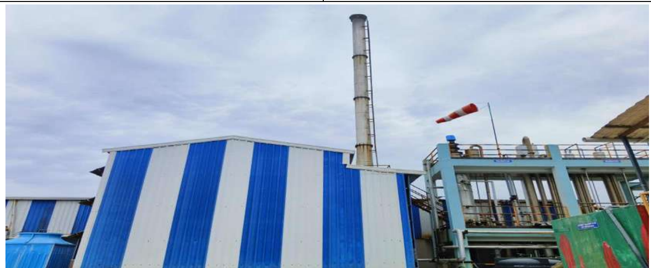
Boiler chimney with stack and dust collector
