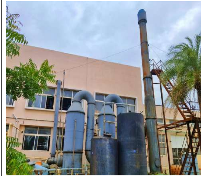
PCMX wet scrubber with chimney
